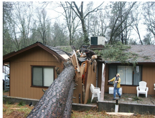
Storm damage - the double-topped pine tree
